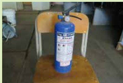
滅火筒 Fire extinguisher
